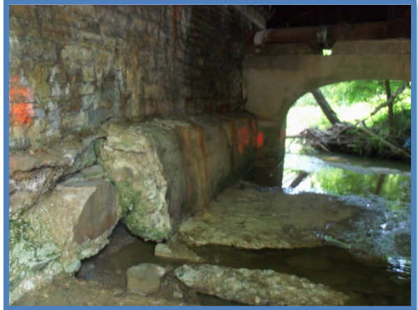
Scour Under East Side of Bridge
